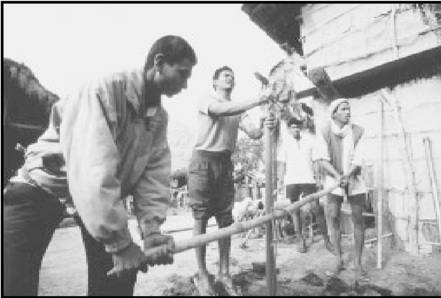
Sinking a tubewell using the sludging method. The work is led by Bipta Chaudray (centre) who is the skilled labourer.
